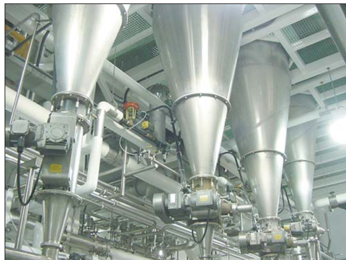
The Briess dryer is housed in a three-story building that is connected to the company's extract plant in Chilton, Wisconsin. The extract plant was commissioned in February 2002 and the dryer was commissioned in March 2005. Both are fully automated, state-of-the-art, food-grade facilities.
